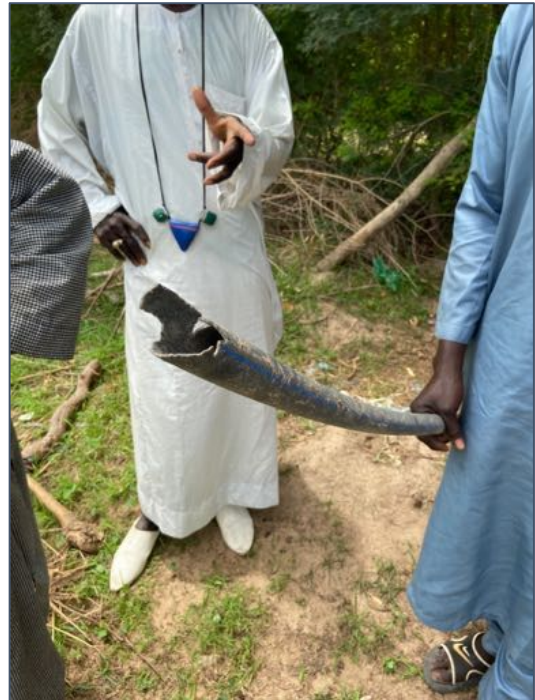
Figure 7: Participants in Medinatou Salame 2 shows the wear and tear in the irrigation pipes.
